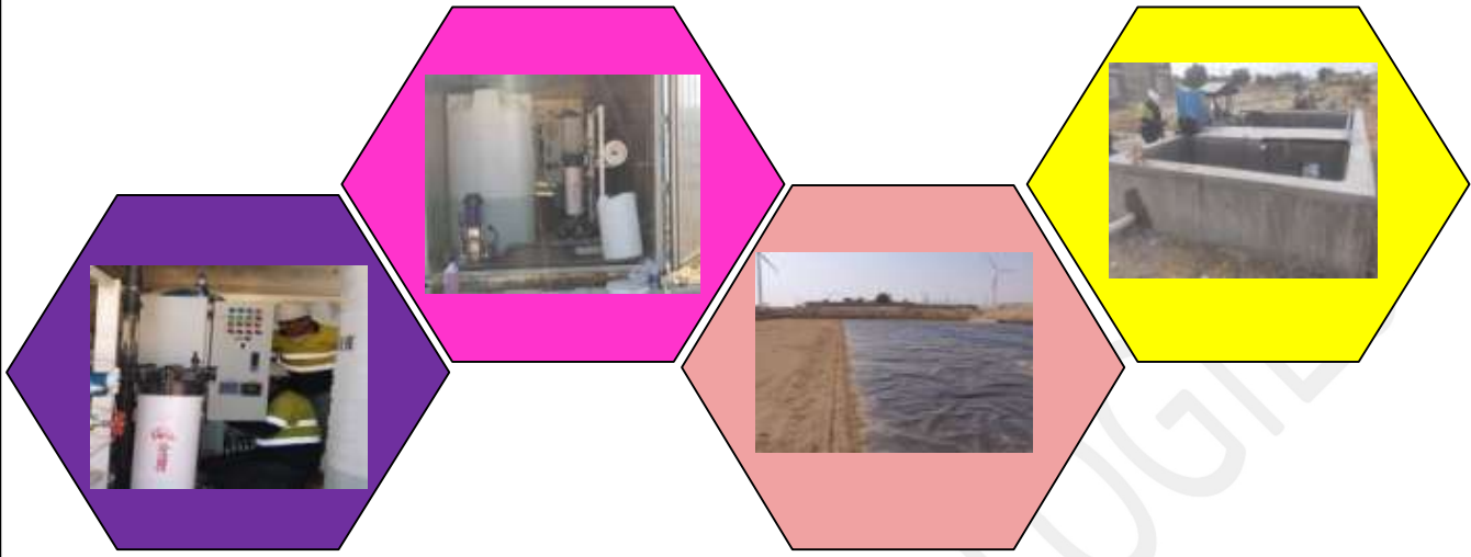
Design and Engineering of 12000 GPD Containerized Reverse Osmosis Plant and STP , Karachi, Pakistan 2018
